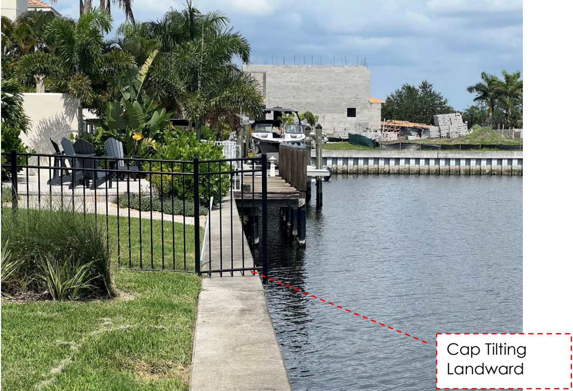
Photo #2- Cap Tilting Landward.
