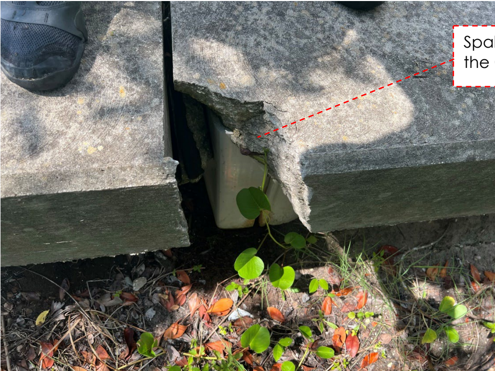
Photo #7 – Typical Spalling of Concrete Cap.
