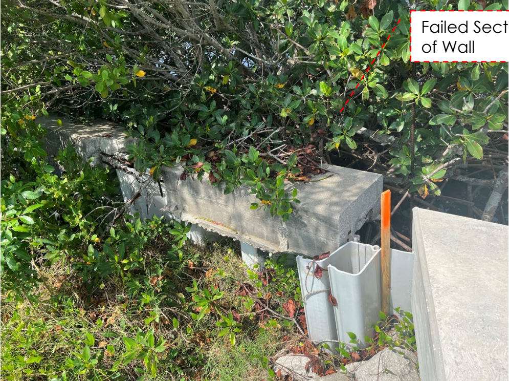
Photo #6 – Failed Section of Wall.
