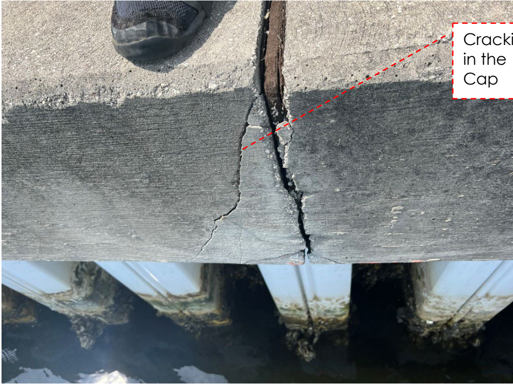
Photo #3 – Cracking in the Cap.
